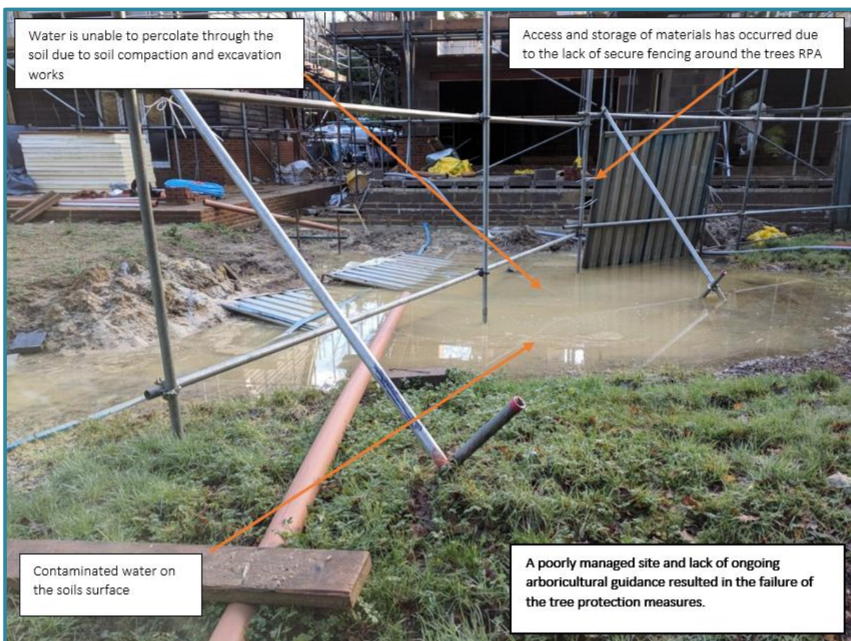
Figure 21. Failure to protect trees to be retained
