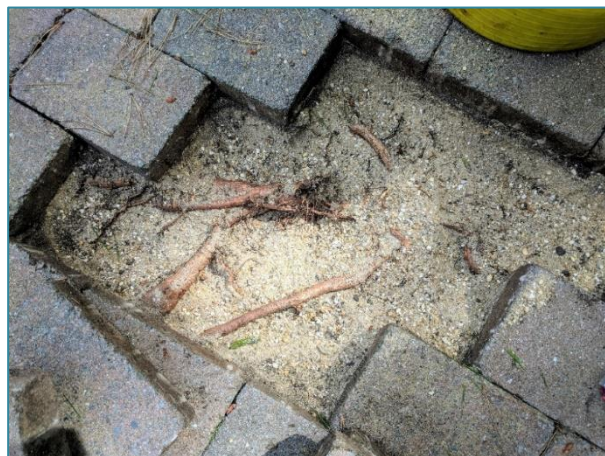
Figure 13. Block paving displacement through root growth and expansion
