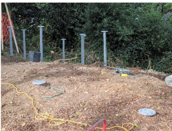
Figure 31. Less invasive screw piles being installed inside the RPA's of protected trees to support new structures
